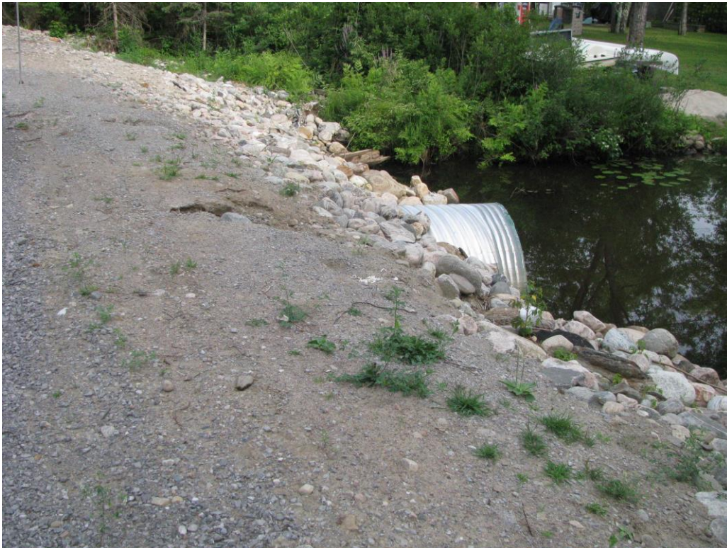
Erosion of exposed soils along the outlet of Merrett Creek, from a culvert installation (Woodworth Drive, July 2016)
